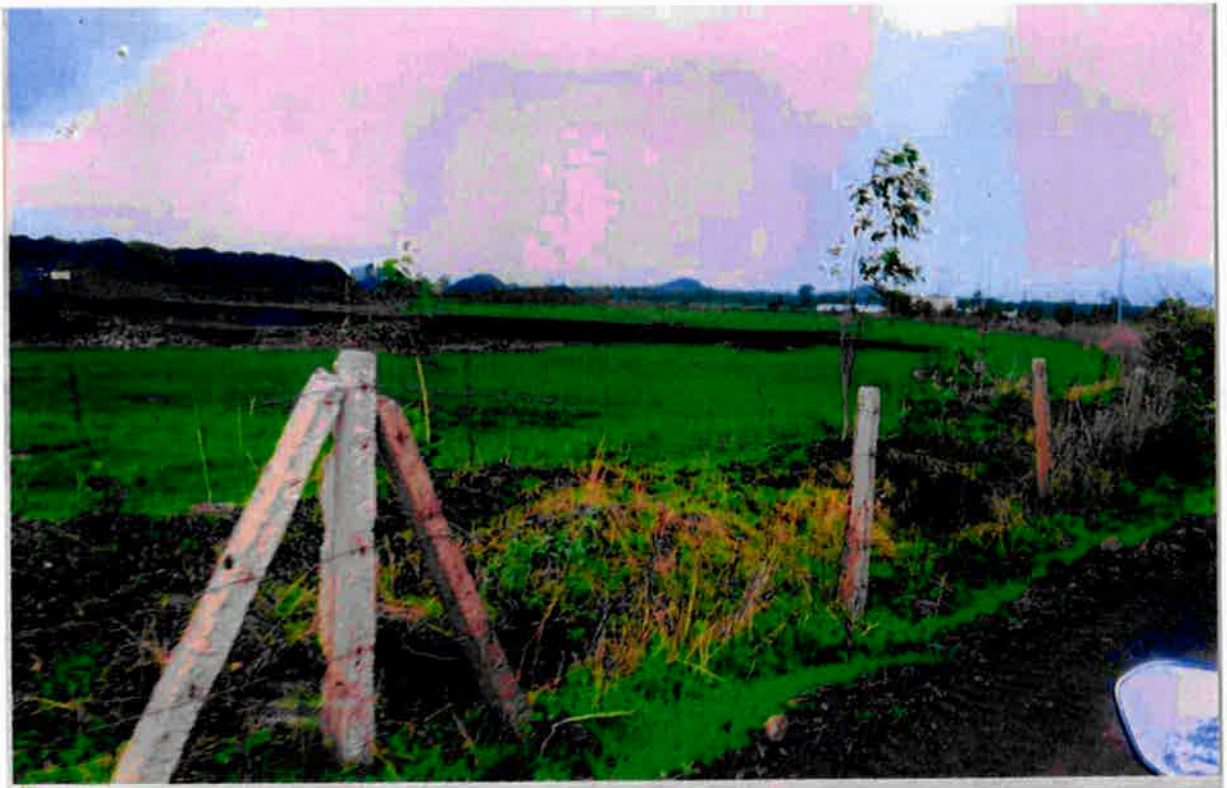
WIRE FENCING AROUND SANCTIONED QUARRY LEASE TO AVOID RISK OF ACCIDENT
